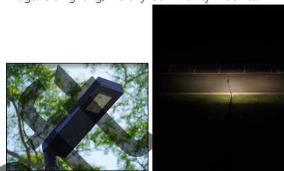
Image: New luminaires at Maleny Community Precinct.
